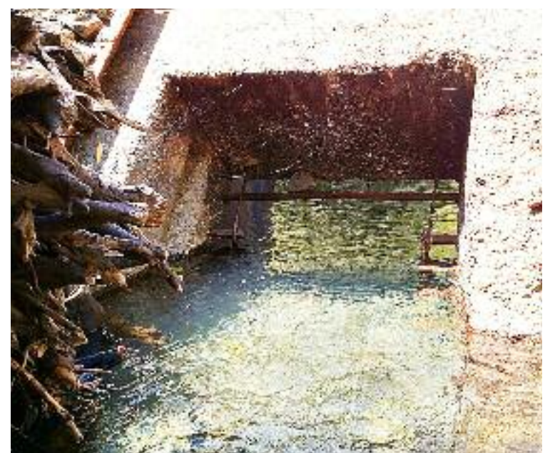
The opening in the drop structure on upper San Pablo Creek unexpectedly blew out last fall, which would have allowed fish to migrate up into its native waters. The opening is clogged again.
